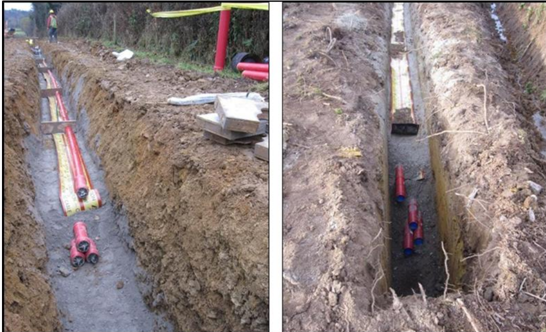
Plate 4-7 Typical Cable Trench View
