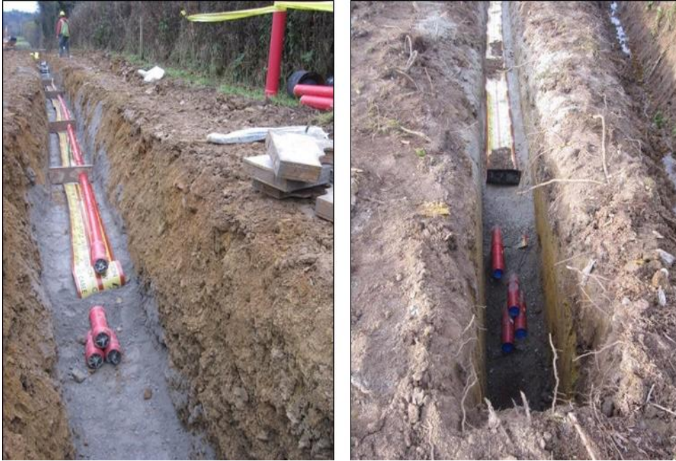
Figure 2-4: Typical Trench Cable View
