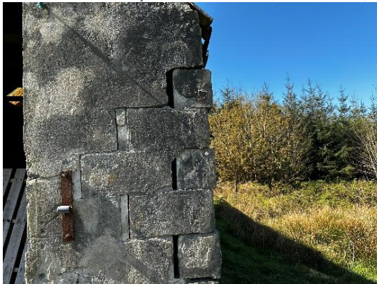
Plate 4-16 Gaps within stonework of Farm Shed A (Structure No. 2)
